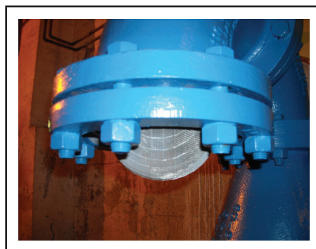
VentSafe® Security Cage Installed on Vent Pipe
